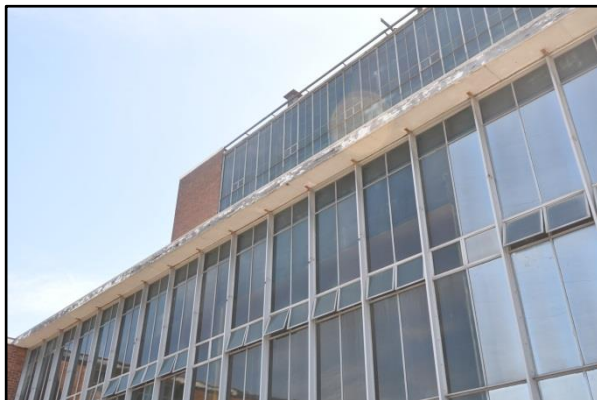
Figure 41. View of clerestory aluminium glazing as viewed from the second-floor roof space.
